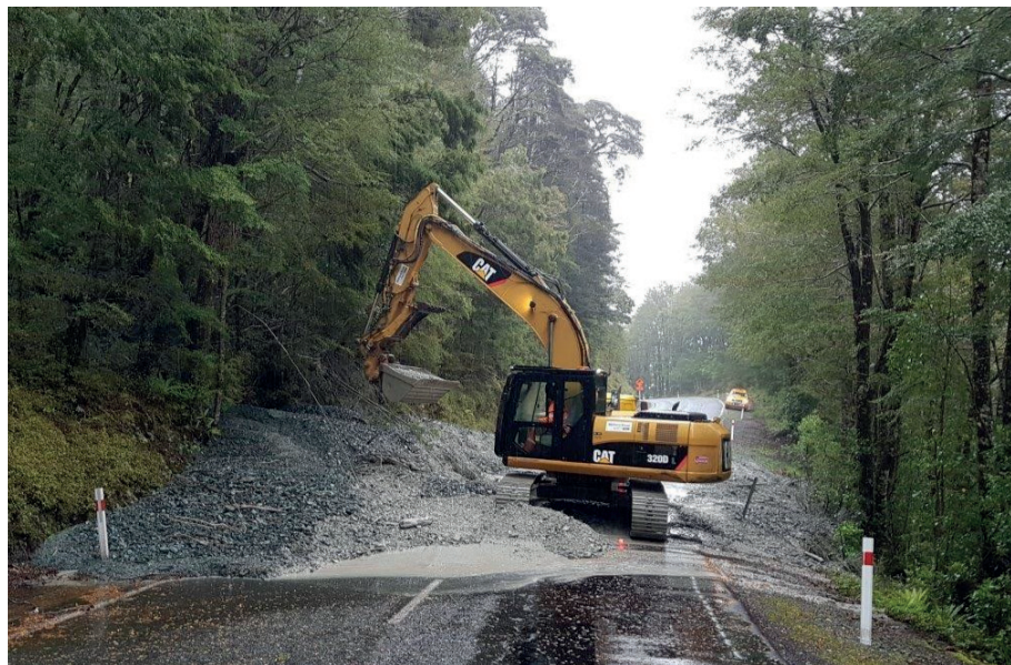
Heavy rain can scour loose rock and bring down slips like this on to Milford Road.
