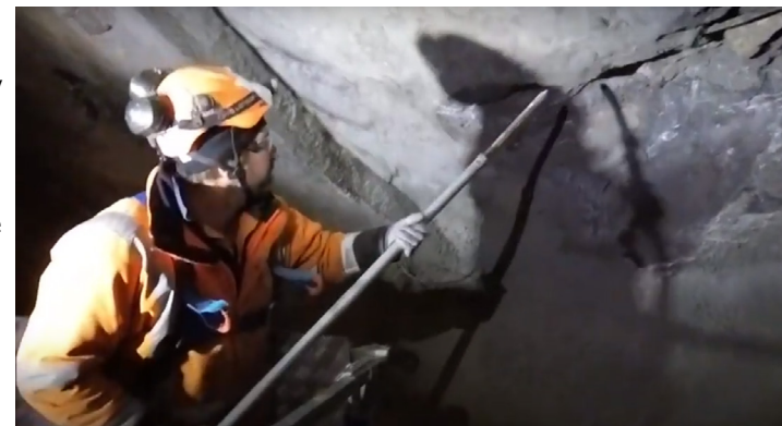
Removing loose rock from a section of wall inside the Homer Tunnel
