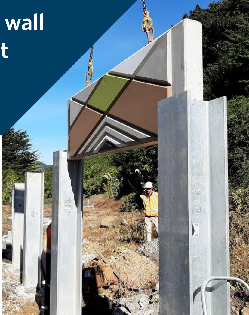
One of the first retaining wall panels complete with local artwork is lowered into position at the Roseneath cutting.
