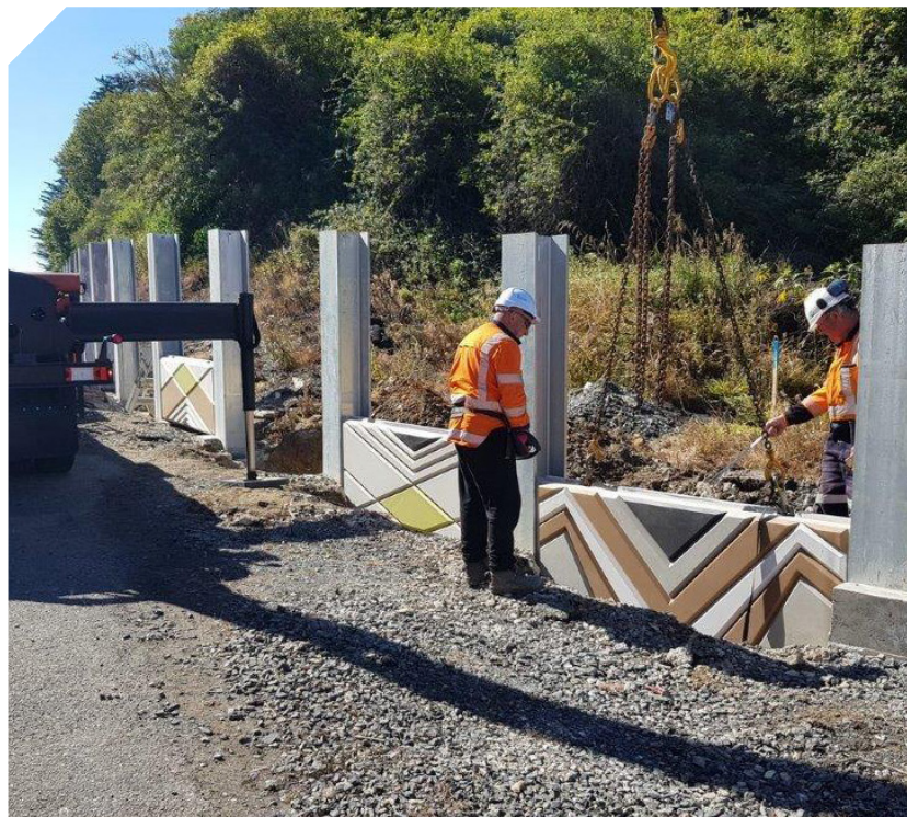
The first of nearly 130 retaining wall panels that will be placed by April/early May at Roseneath to support the new Dunedin to Port Chalmers shared path.
