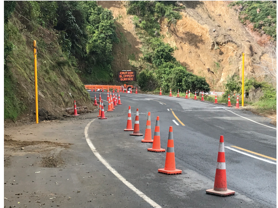
The poles to support traffic signals being installed on Takaka Hill road in recent days.
