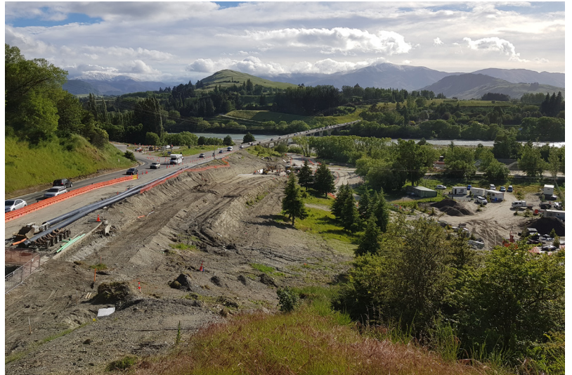
Good progress is being made on the formation of the new slip road
