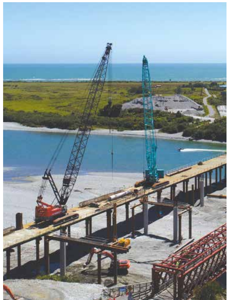
Large cranes based on the temporary bridge are being used to get piling equipment in and out of the riverbed
