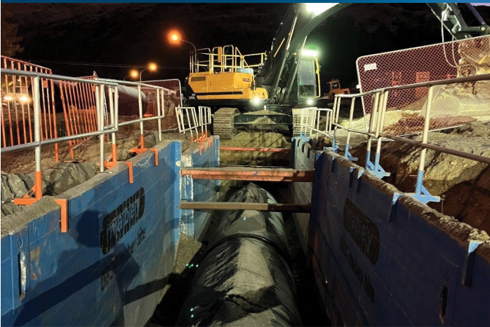
This pipe provides a stormwater outlet for the new layout at the Frankton intersection
