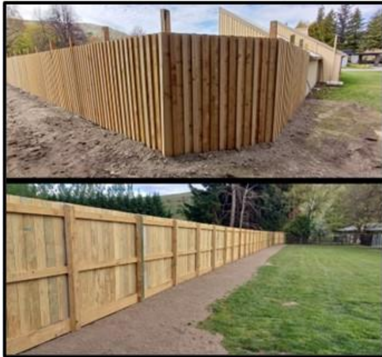
The new fence built at the Ladies Mile Pet Lodge, completed in time for holiday bookings.
