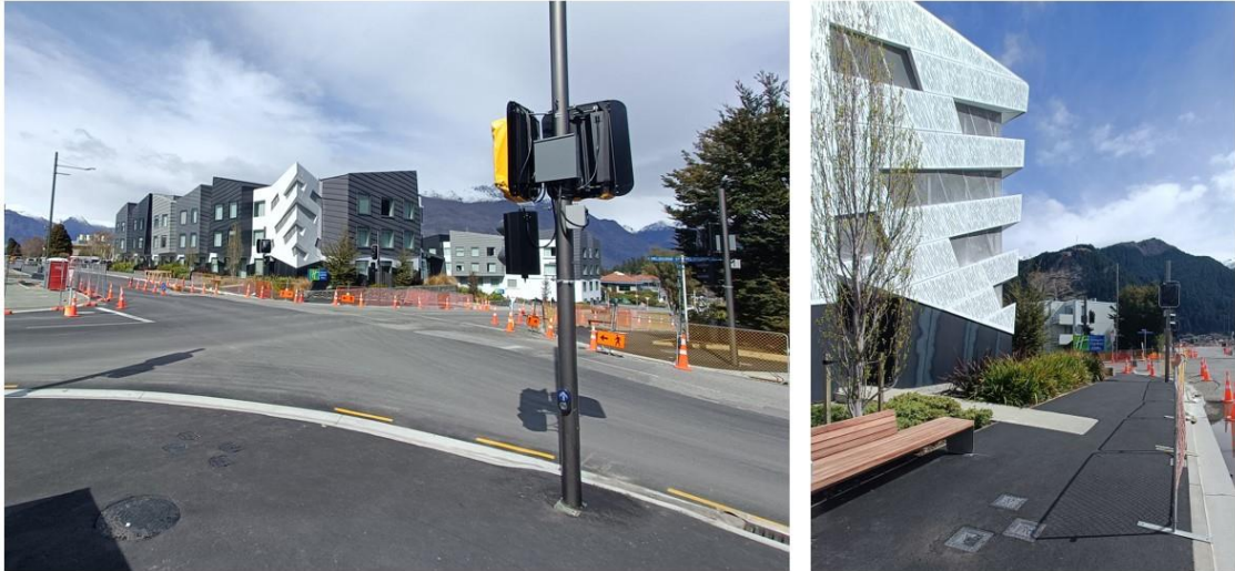
(Left) We will soon begin work on the lower side of the Sydney-Melbourne intersection, due for completion by the end of October, and (right) completed footpath on lower Sydney Street.
