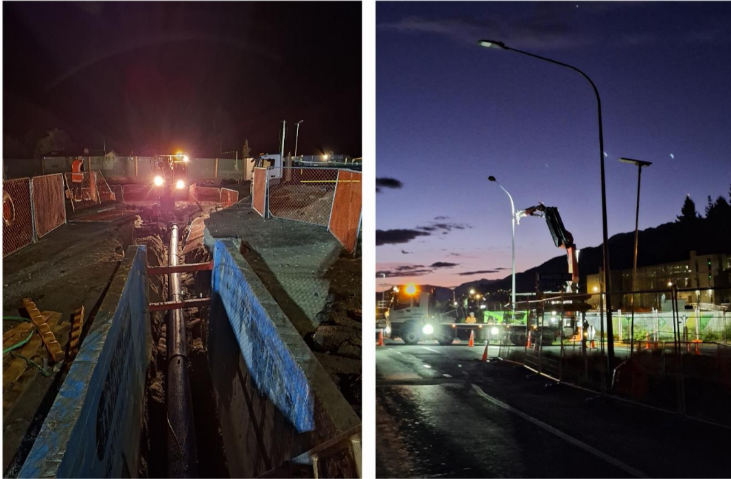
Left, the new drinking water pipeline connected in place, and right, the team temporarily relocates a light pole in order to excavate a foundation for its permanent position.
