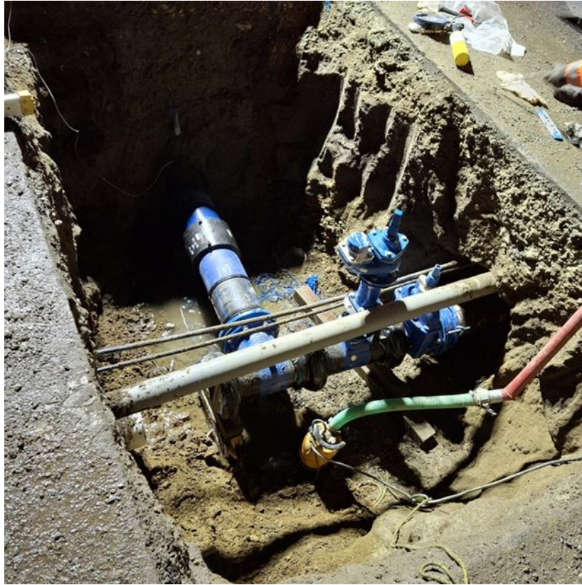
Part of the new water supply system for Frankton, built as part of the Queenstown Upgrade.
