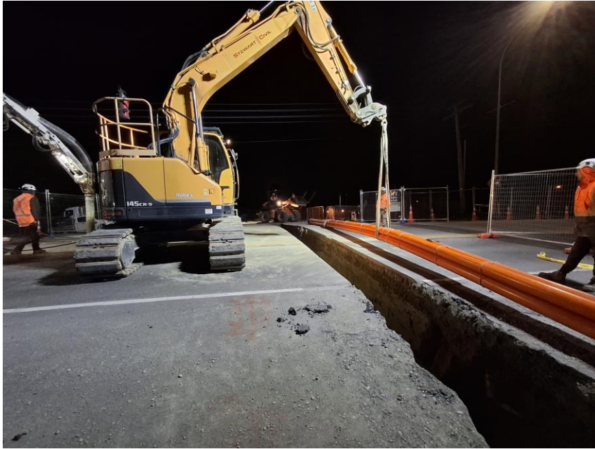
Precise trenching across the state highway, helped by no rain or wind.
