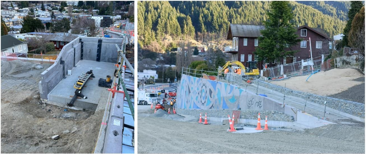
Left, our team building the stairs connecting Melbourne and Beetham Streets, and right, the pedestrian ramp between Ballarat and Henry Streets.
