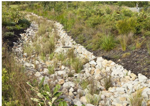
Rock lined stormwater infrastructure with native grass mixes
