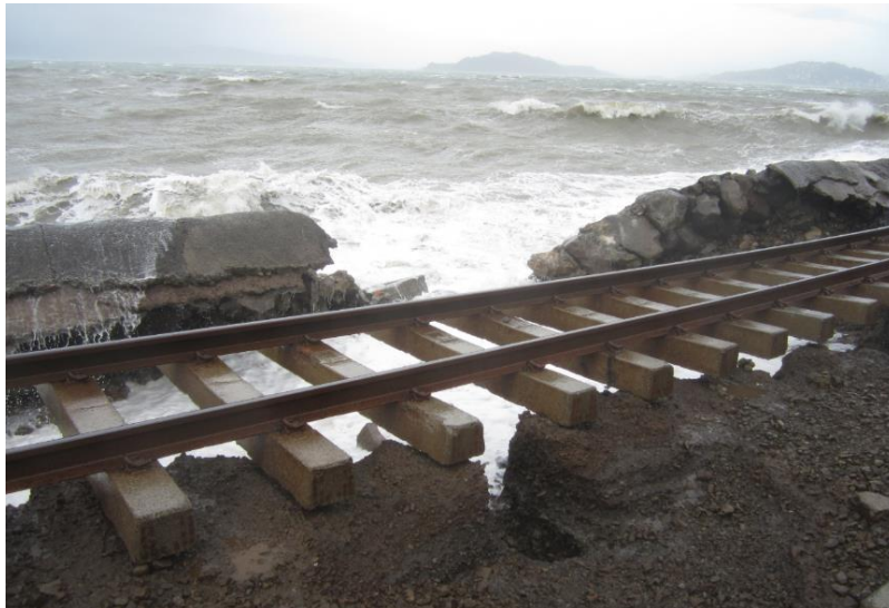
Figure 5 Wash out of the Hutt Valley Rail Line in 2013
