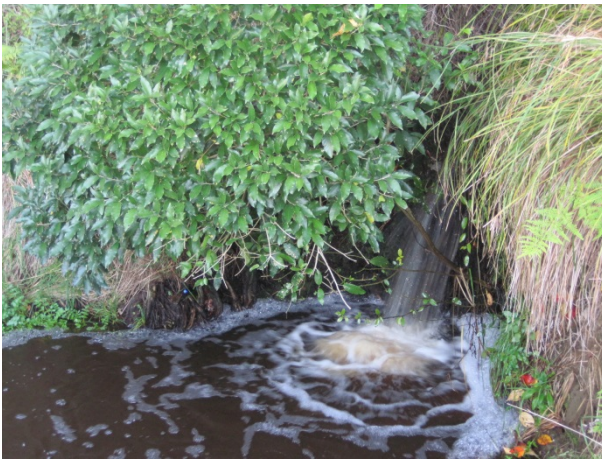
Figure 3-17: A perched pipe is present on Stream 2 beneath SH1 (within Designation)
