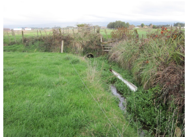
Figure 3-18: Downstream of the Designation a second perched pipe is present on Stream 2
