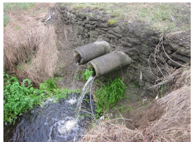
Figure 3-20: Stream 3 (within Designation) is fed by two perched pipes beneath SH1
