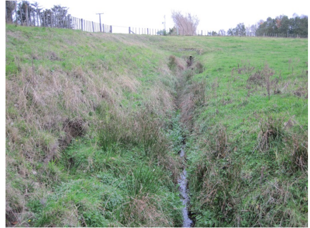
Figure 3-29: Mudfish were present in the stream closest to SH1 with less stock damage
