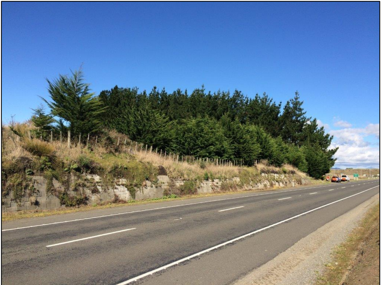
Figure 3-1: Pre-existing large concrete block retaining wall placed to stabilise sand dune slope cut adjacent to SH1.
