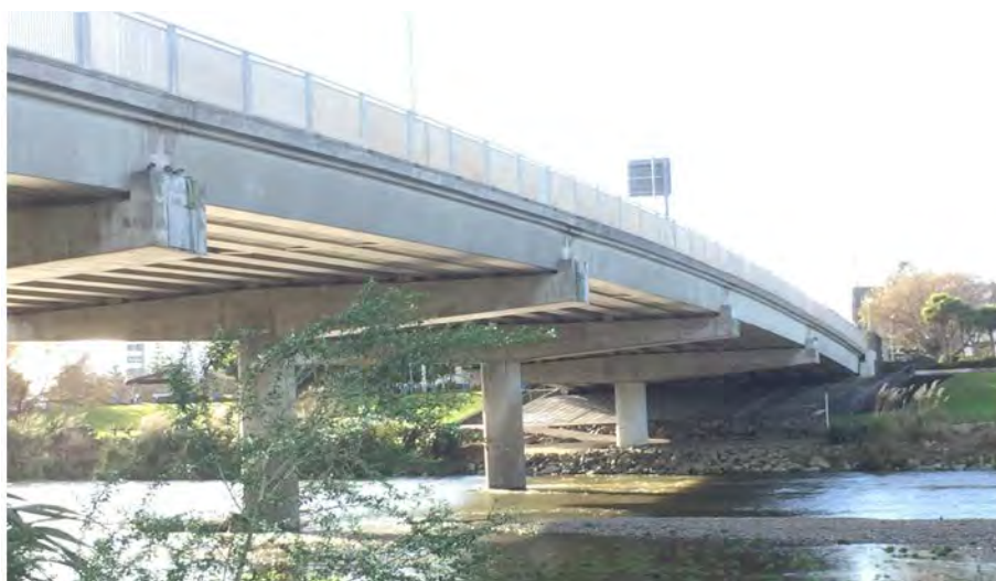
Ewen Bridge showing rock armour and concrete flood and seismic protection measures at the east abutment stopbank
