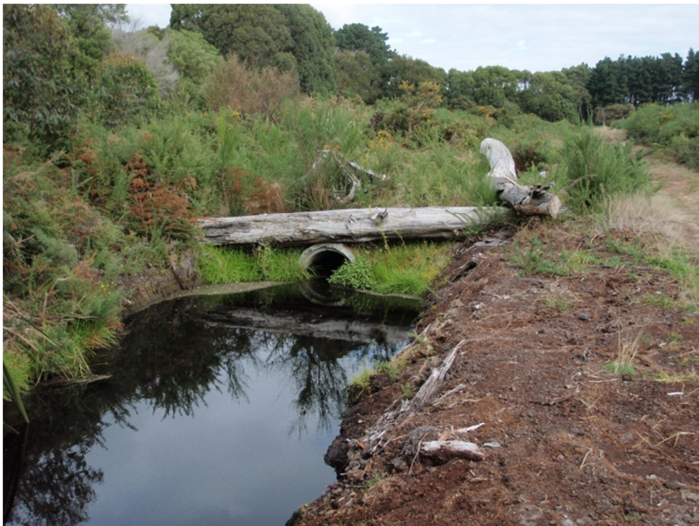
Photo 23 – Upper Drain 7 showing unstable peat dominated substrates in the vicinity of the proposed Expressway alignment.
