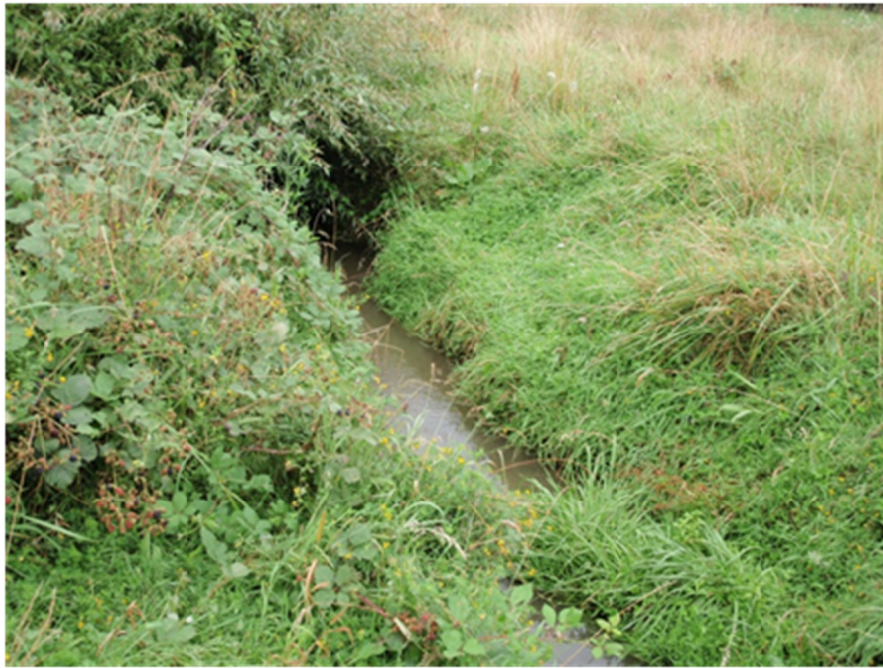
Photo 13 – Muaupoko Stream upstream of walkway culvert, stable stream bank provided by scrub grasses and blackberry.
