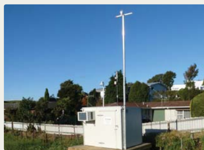
Air quality monitoring station on Raumati Road
