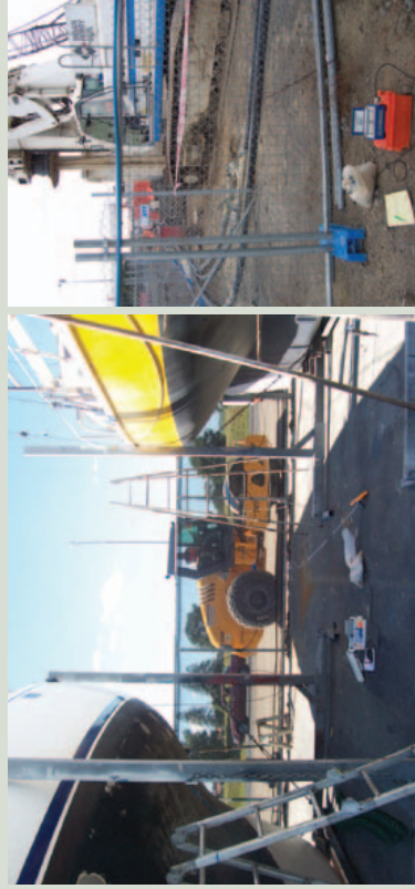
Vibration monitoring equipment PHOTOS: GEOTECHNICS LTD
