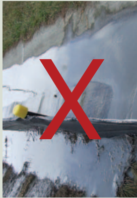
This photo shows uncontrolled discharge caused by poor trenching.
