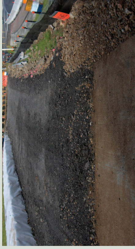
Picture: Stabilised Construction Entrance.
