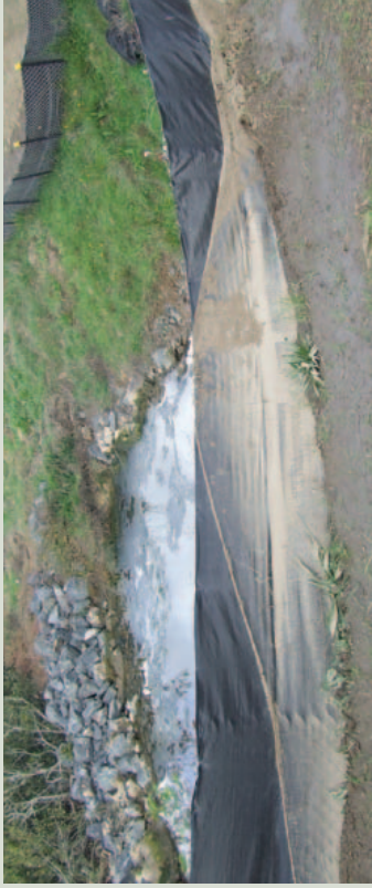
Picture: Silt fence – not level.
