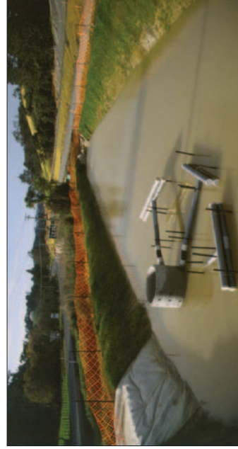
Sediment retention pond (Photo in Auckland region – compliments ARC)
