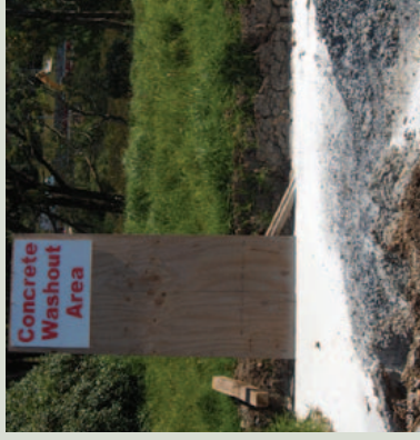
Picture: Concrete washout area. A copy of the sign is available on the CD.
