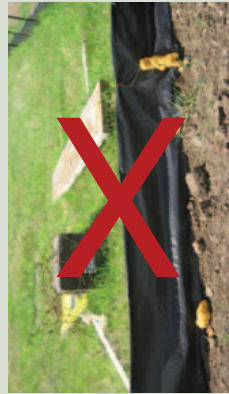
Inappropriate use of Gorilla Filler
