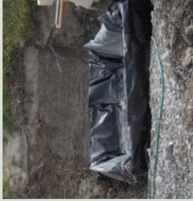
Picture: Polythene lined washout area. Cover when not in use to prevent it filling with rainwater.
