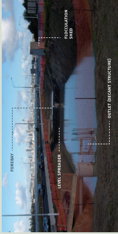
Picture: Typical sediment retention pond.
