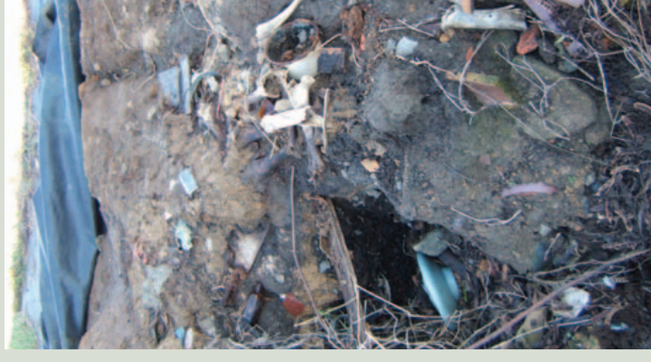
Picture: Old fill site located within new road alignment.
