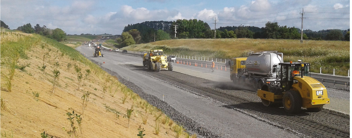
Hi-lab pavement work under way on the new north-bound lanes near the Te Kauwhata interchange.
