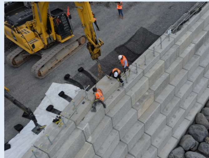
OCTOBER Last sea wall block for the whole project placed at Half Moon Bay
