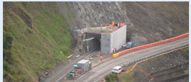
Tunnel 13 just south of the Kahutara Bridge is being transformed by the hard work of the tunnel crews involved.
