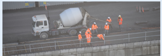
Crews are pouring concrete for the shared path at Ōhau Point north of Kaikōura – this will also act as the capping beam for the seawall. This is the location of one of the massive slips that cut off Kaikōura from northern access to State Highway 1 last year.
