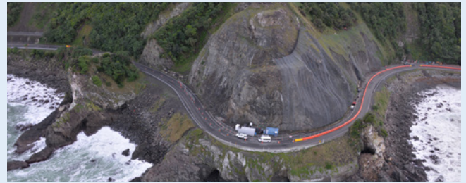
The crown of mesh adorning the Punch Bowl helps to prevent rock fall and slip movement, keeping the road below safer for travellers.
