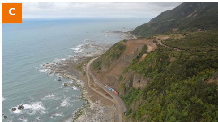
The flat work site at the top of the slip is clearly visible from this angle.
