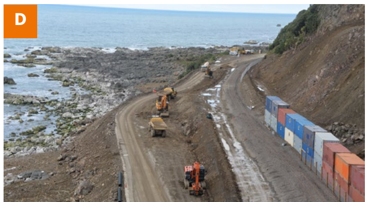
Work is well underway on the road realignment around the toe of the slip. The construction access track is also being widened to two lanes.
