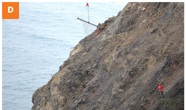
Abseilers working to secure rock mesh netting high up on the north face of Ohau Point.
