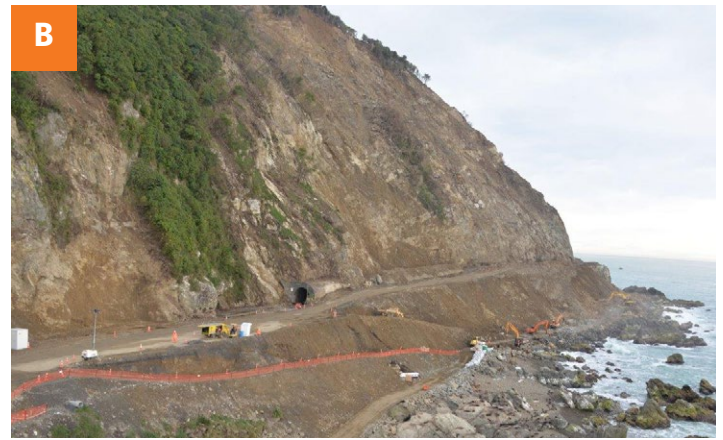
The south side of Ohau Point has been slliced, scaled and an access track is being built around the outside of the point for construction traffic.
