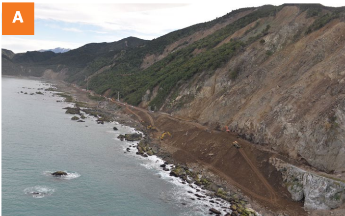
Photo showing the extent of work done to date on the road south of Ohau Point.
