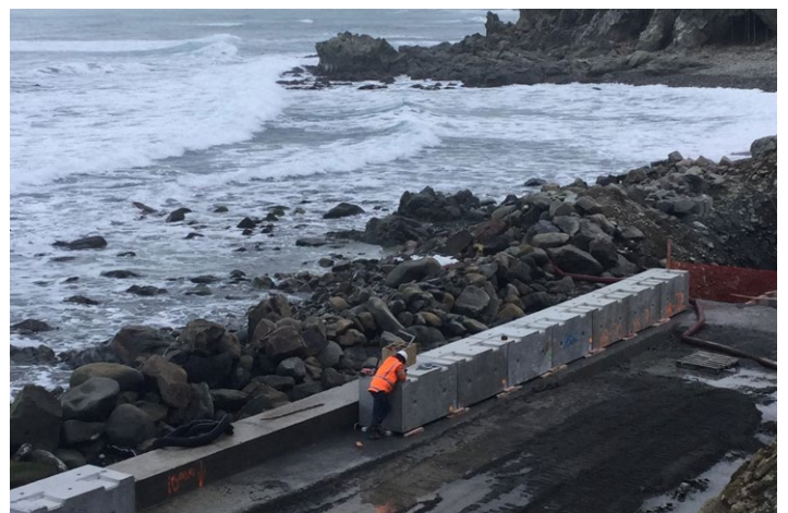
Milestone: The first of the seawall blocks were laid at Site 2 near Irongate this week.
