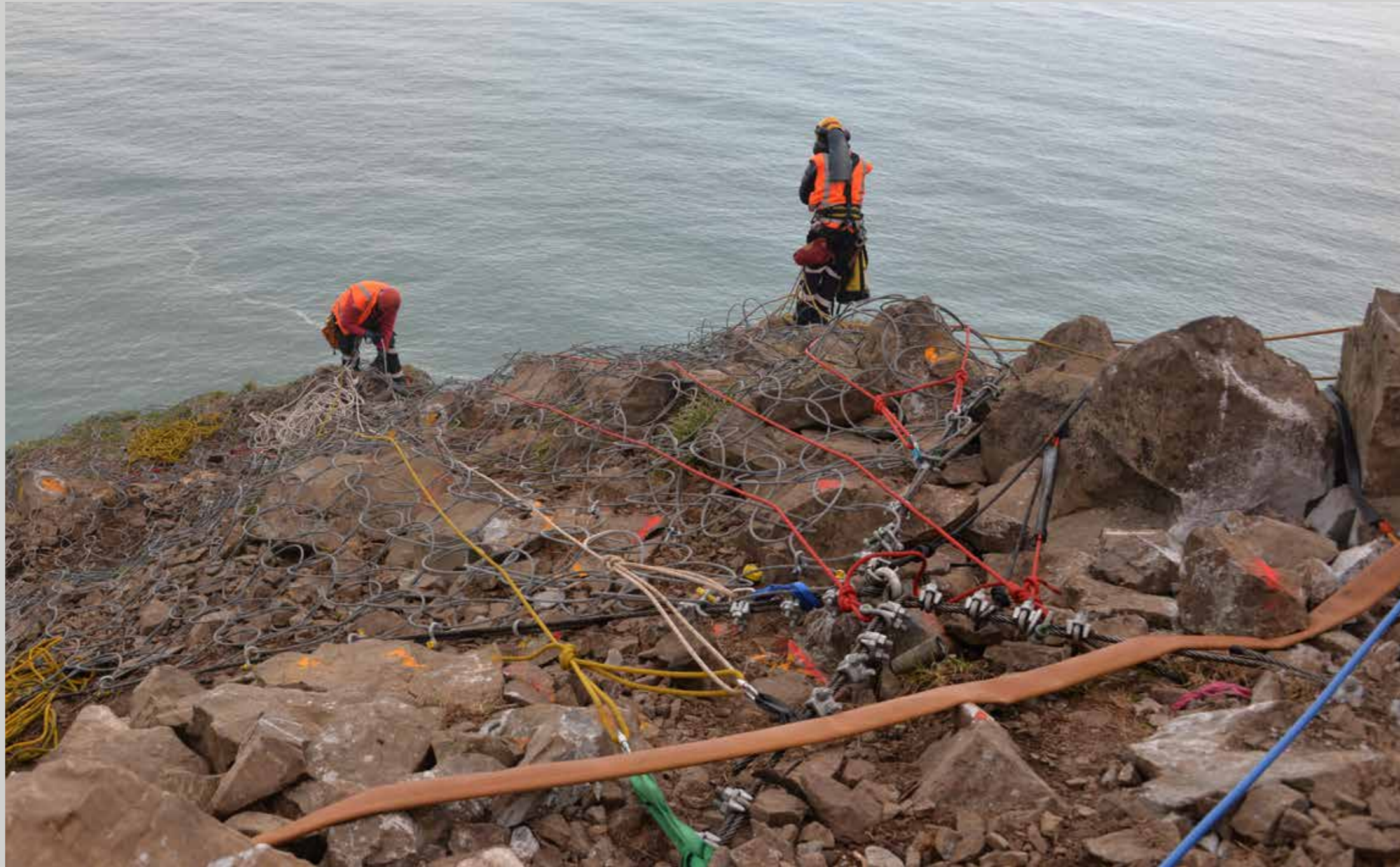
Response to Rebuild
