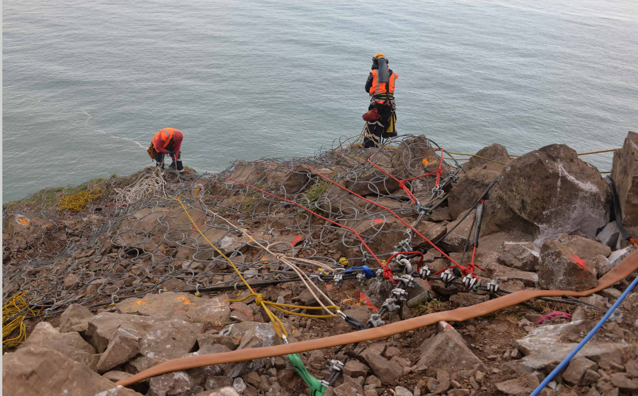
Response to Rebuild
