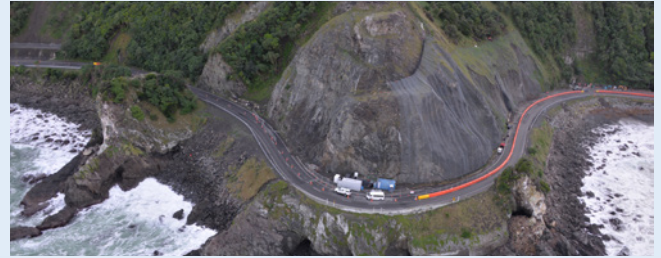
The crown of mesh adorning the Punch Bowl helps to prevent rock fall and slip movement, keeping the road below safer for travellers.
