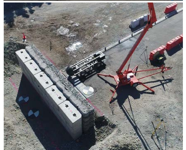
Standing proud as the new modular rockfall protection wall holds up in testing.
