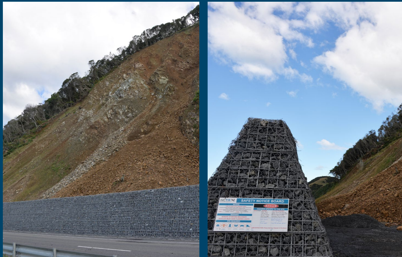
At Site 1 near Mangamaunu a new gabion basket rockfall protection wall stood up strong, on one side sat an untouched road and rail line, and on the slip side, fresh material was piled up ready to be collected and removed.
