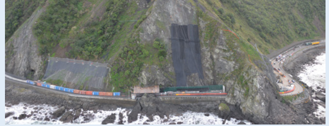
While traffic flows south of Kaikōura, work continues at Sites 16 and 17 above the Parititahi Tunnels, and at Sites 18 and 19, south of the tunnels.
