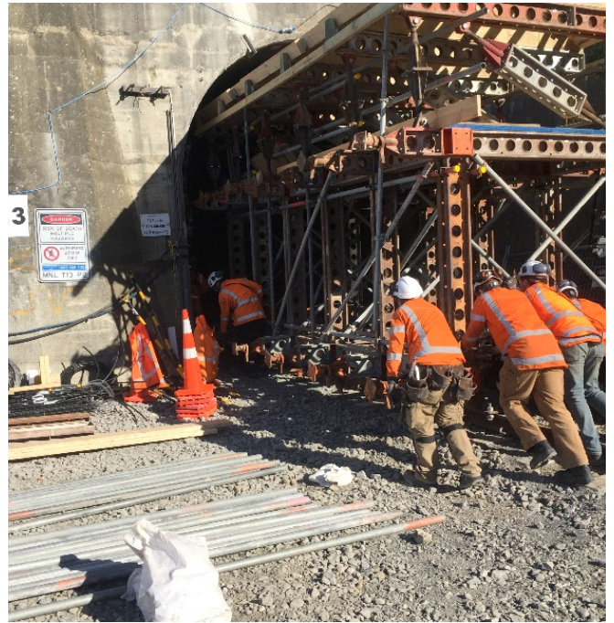
Safety first: The tunnel propping system can be rolled into place to keep tunnel repair workers safe.
