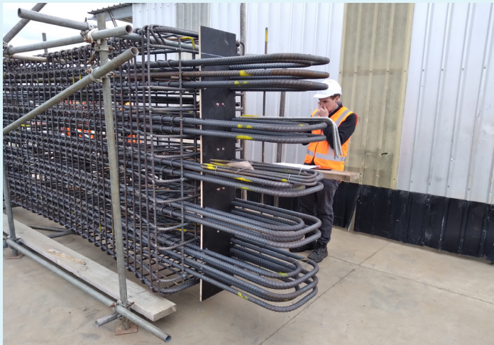
Some of the steel reinforcing rods for the precast concrete modules for the new rockfall shelter.
