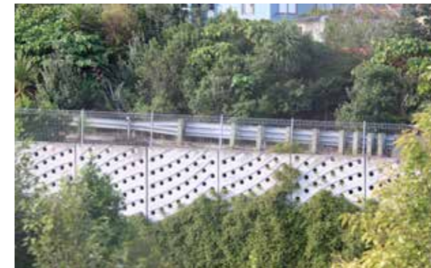
Integrated planting design (Hobsonville Rd / SH16) - climbers where space in front is limited
