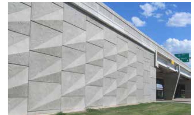
Southern Motorway, Christchurch - pattern of light and shade visually breaks down large walls
