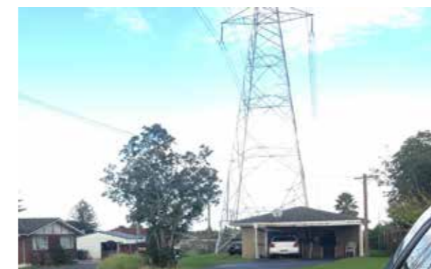
Transmission towers in Panama Road area
