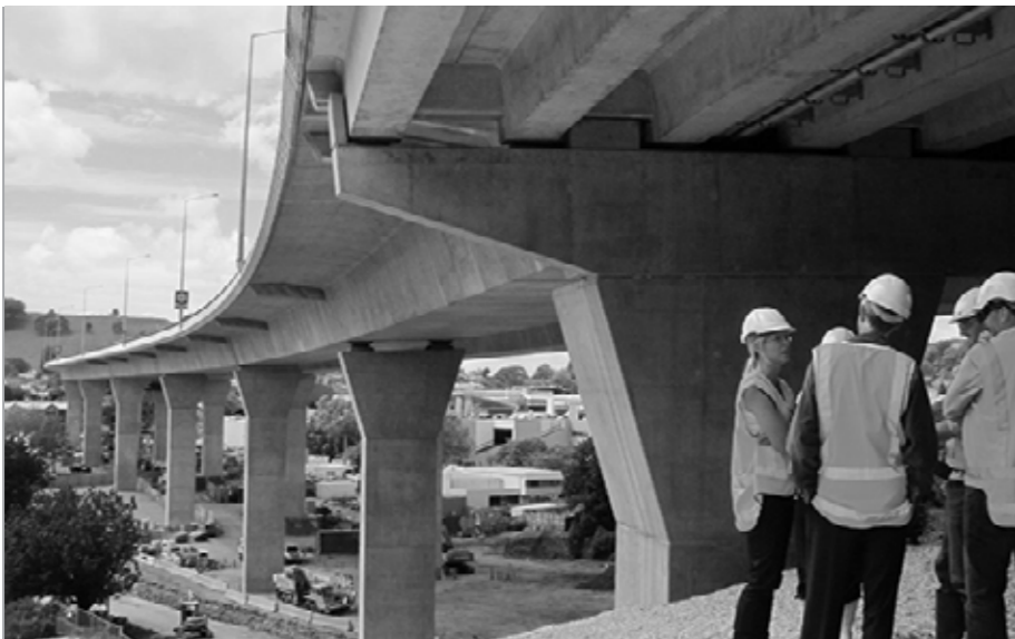
Newmarket viaduct - parapet design results in a fine horizontal line through the landscape
