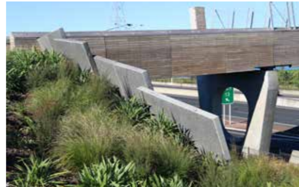
Onehunga Bay Foreshore pedestrian bridge - a combination of vertical and sloped abutments, and sculptural piers, is a strong feature and creates a good under-bridge environment for the motorway and path network
