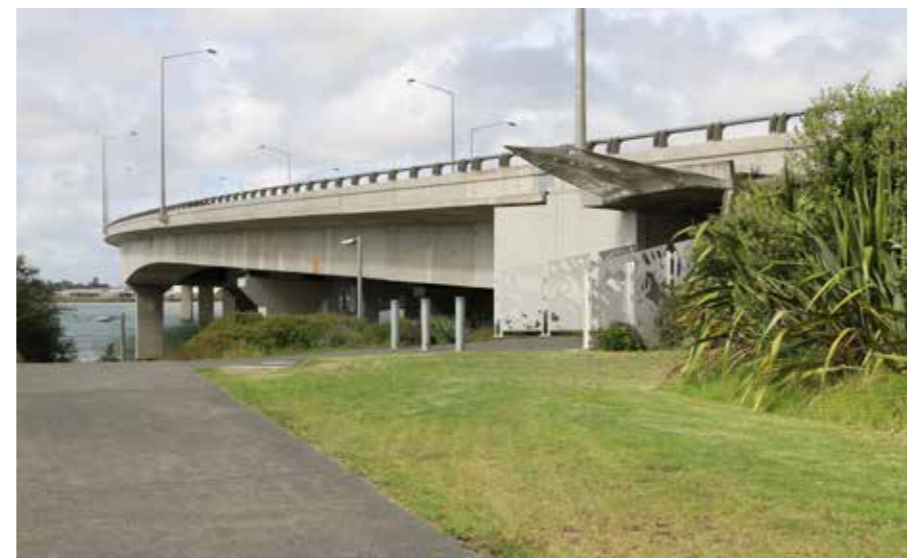
Lower Onehunga Mall / SH20 Underpass: a change of direction is signalled by the entry portal / decorative screen to improve the approach
