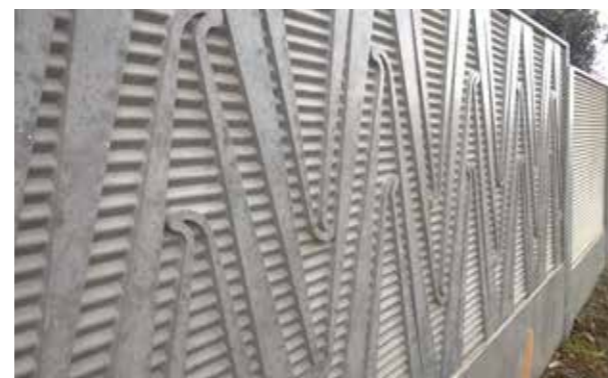
Kirkbride Road / State Highway 20, Auckland - fine detail on noise wall alongside shared path
