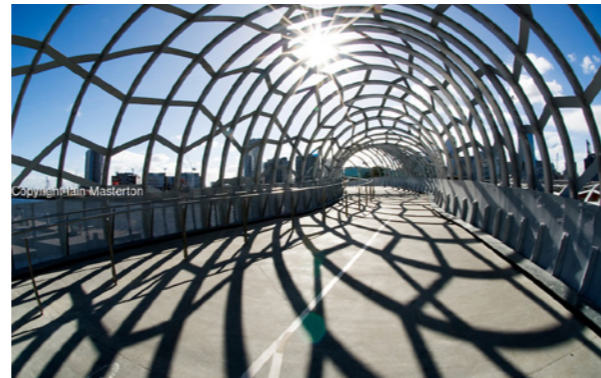
Webb Bridge, Melbourne - re-use of materials to create a unique sculptural form and experience
