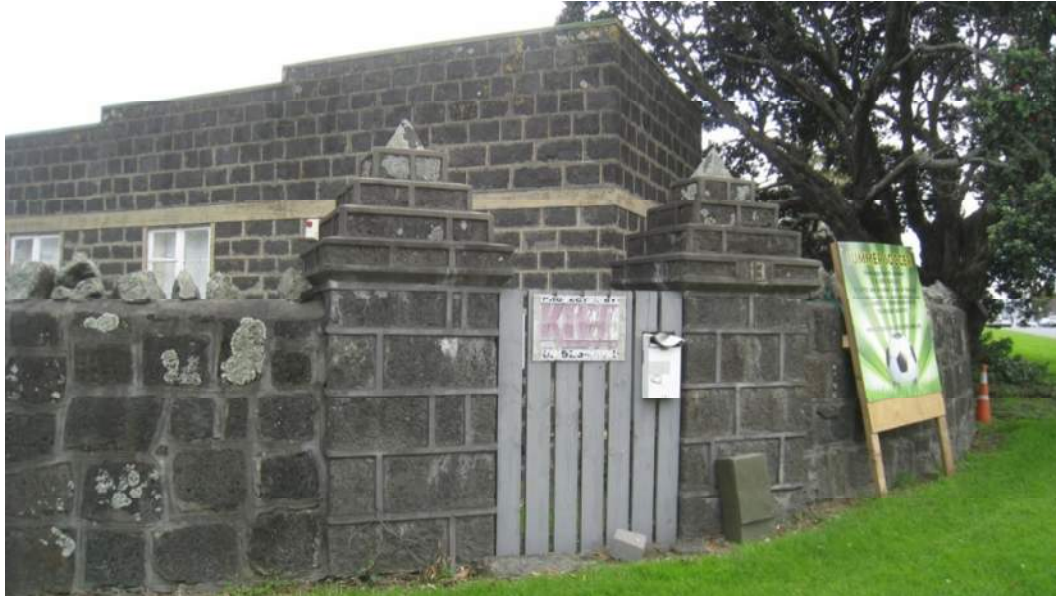
Figure 5-13: Stone walls, piers and Caretaker’s Cottage, Waikaraka Park, at corner of Captain Springs Road. Photo Matthews & Matthews Architects Ltd, September 2016.
