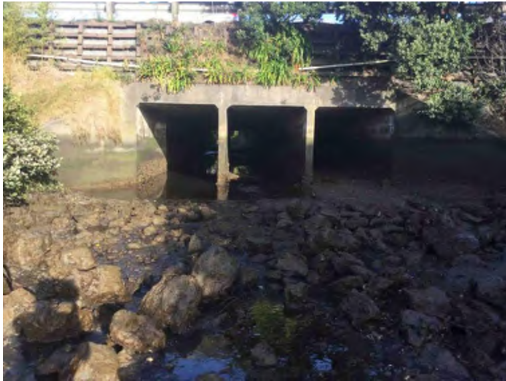
Box culverts under SH1, upper Otahuhu Creek.
