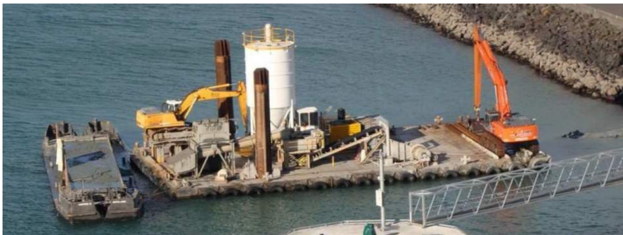
Figure 7-6: Typical marine based mudcrete plant
