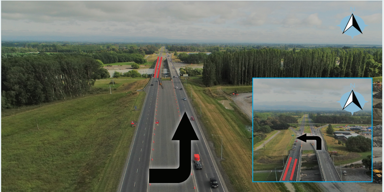
A temporary sealed section of road at the southern and northern end of the Waimakariri Bridges accommodates the contraflow: on Sunday night 3 February traffic on the closed northbound bridge takes the southbound bridge to cross.
