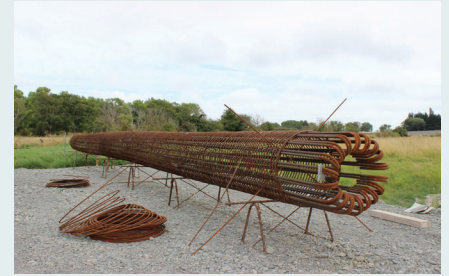
Part of the steel reinforcement that will be placed in the steel casing to fill with concrete.
