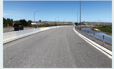
The work to four lane QEII Drive between Main North Road and Innes Road will be completed in June 2020.
