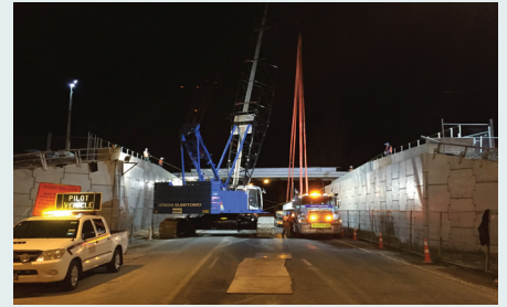
Placing the beams for the Main North Road Bridge (a similar night time operation will occur at QEII Drive overbridge, planned for February 2020).
