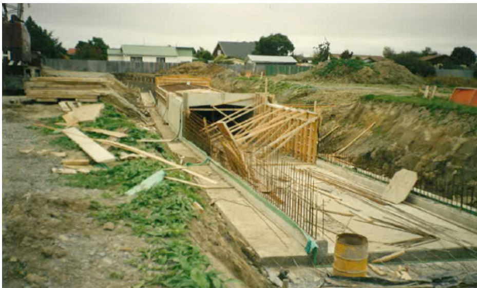
Building the Grimseys Road subway December 1994 – photo supplied by Helen who lives on Grimseys Road.
