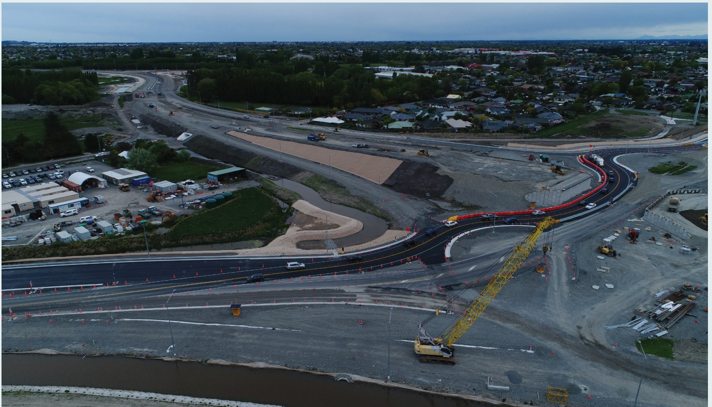
TRAFFIC WAS MOVED ONTO THE SOUTHERN HALVES OF THE NEW QEII DRIVE ROUNDABOUTS.
