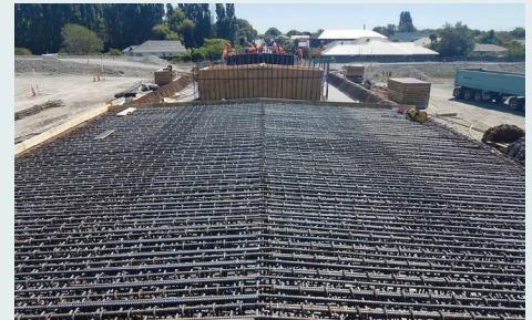
135t of reinforcing steel was used within the concrete so it can carry the weight of the new motorway on top of the subway roof.
