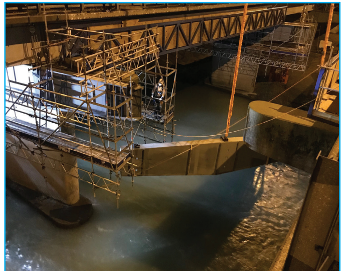
Lifting the steel headstocks in place at night. These headstocks are mounted on the piers to strengthen them so they can carry the bridge spans and new deck.
