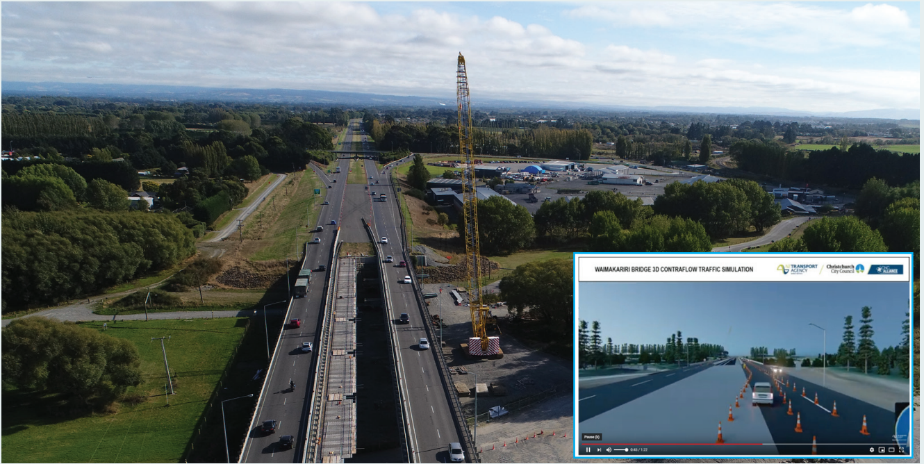
A temporary sealed section of road at the southern and northern end of the bridges accommodates the contraflow. An animated video on our website: www.nzta.govt.nz/cnc shows how the Waimakariri Bridge contraflow will work.
