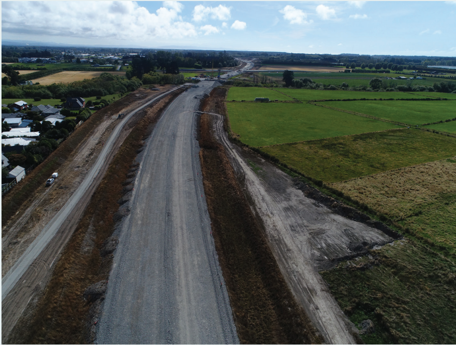
Looking north to the Styx River bridge location. Left of the motorway is the shared use path in construction.
