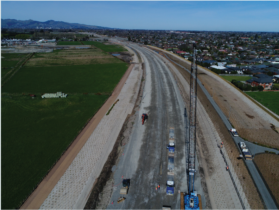
Looking north from the Styx River bridge to the right of the motorway is the shared use path in construction.
