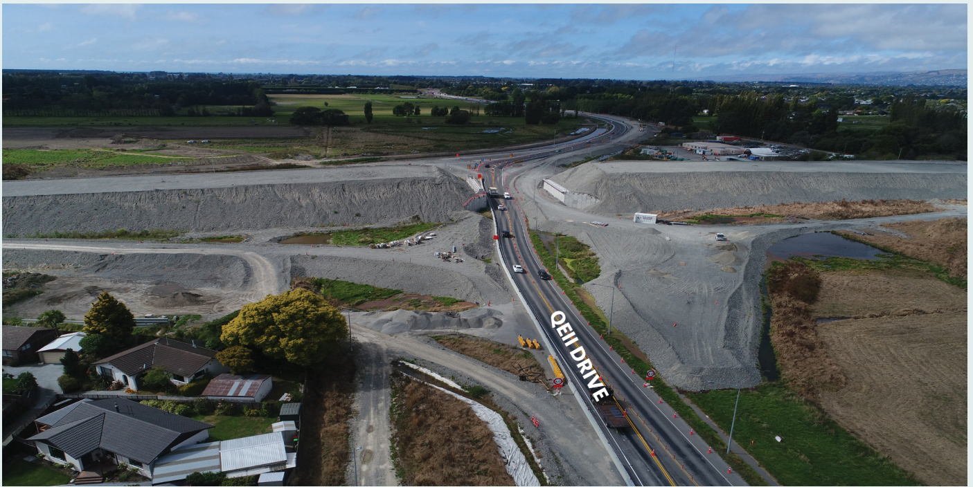
The new CNC motorway goes over QEII Drive on a bridge. Two roundabouts connect the traffic coming off the motorway to QEII Drive and leaving QEII Drive to connect to the motorway going north or south to Cranford Street. For more information on our structures watch the videos on our website: www.nzta.govt.nz/cnc
