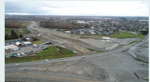
Aerial view of the QEII Drive interchange, with the new CNC motorway going over QEII Drive (bridge walls are visible).
