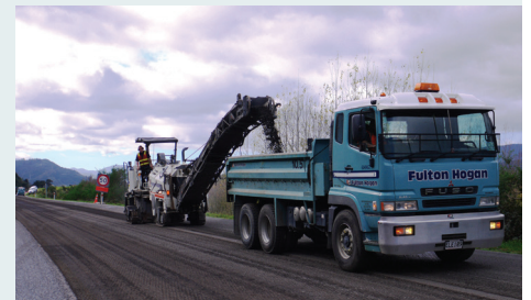
Milling the road will be noisy. Please take care around the work site during the surface work.
