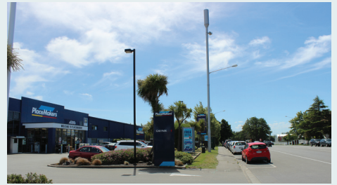
Please support the businesses on Cranford Street and continue to shop local during our works.
