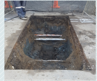
A trench showing underground services. We will have to relocate the power and telecommunication cables.
