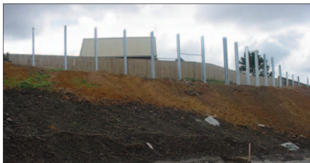
Some of the noise barriers on the Greenhithe deviation project in Auckland have been designed so they can be increased in height at a future date
