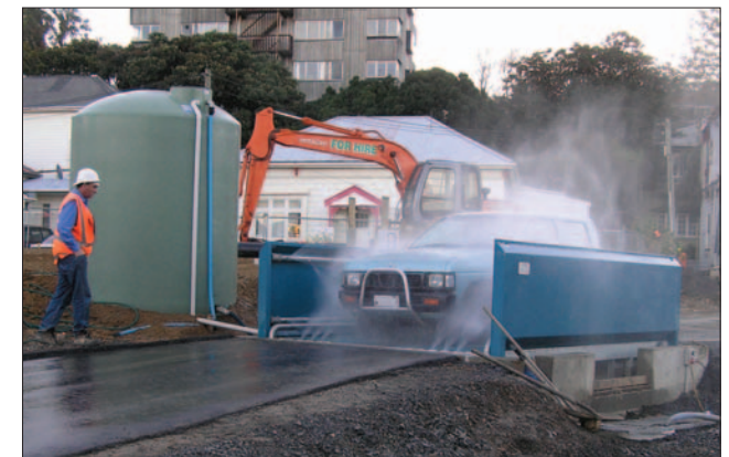
Wheel wash facility used to control dust from the Wellington inner city bypass project
