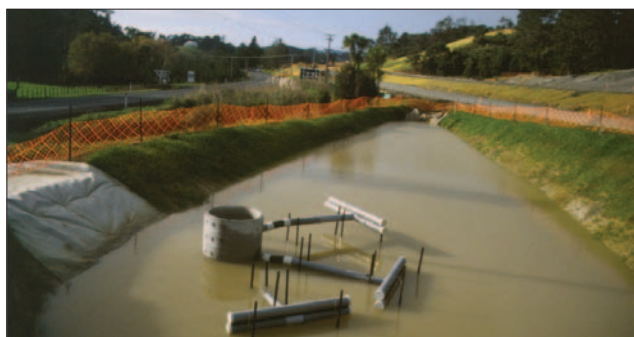
Sediment retention pond (Photo in Auckland region – compliments ARC)
