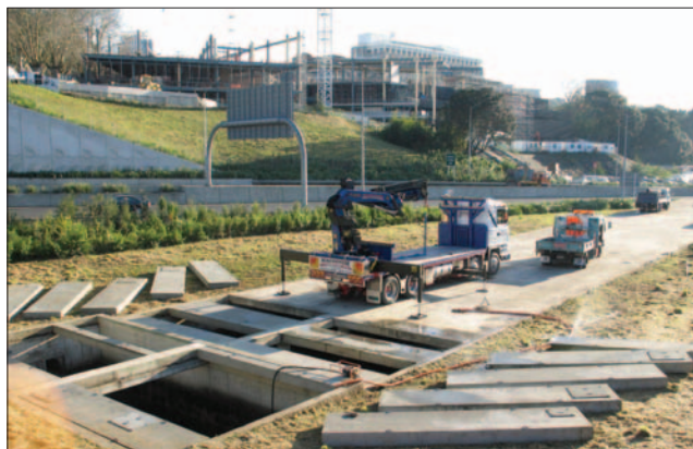
Grafton gully stormwater and spill retention tank
