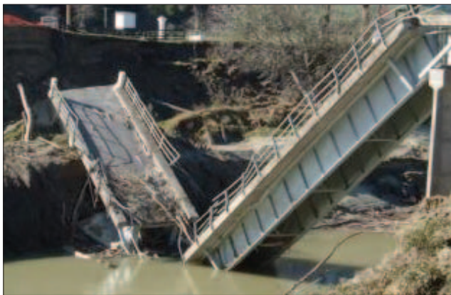
Flood-damaged bridge, Wanganui
